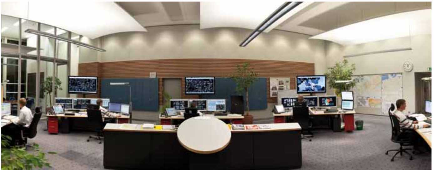
Control room in Dachau
