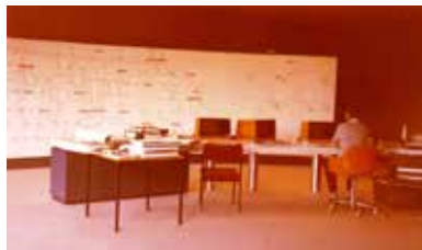
Electrical energy control room at Stadtwerke Aachen 1973.
