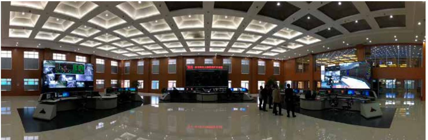
The PSImining control room at Shendong.
